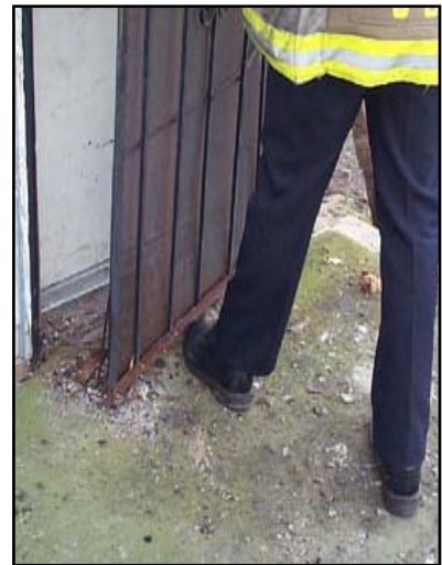
Photo 6: “Footing” the door will prevent a sudden loss of balance.
