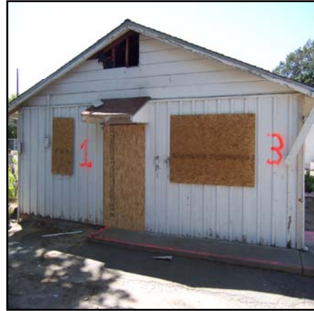
Photo 11- Clearly mark the burn rooms according to the Incident Action Plan.
