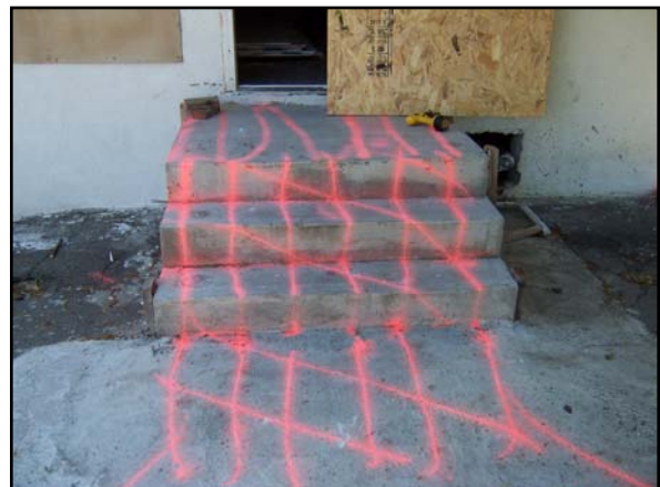
Photo 9- Clearly mark all hazards, including steps.
