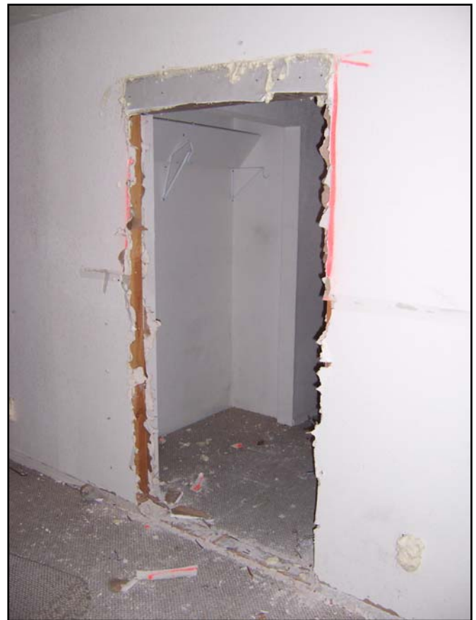
Photo 14- Adding doors through walls can provide different paths for fire attack..
