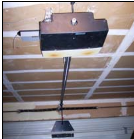
Photo-3: Typical electric garage door opener.
